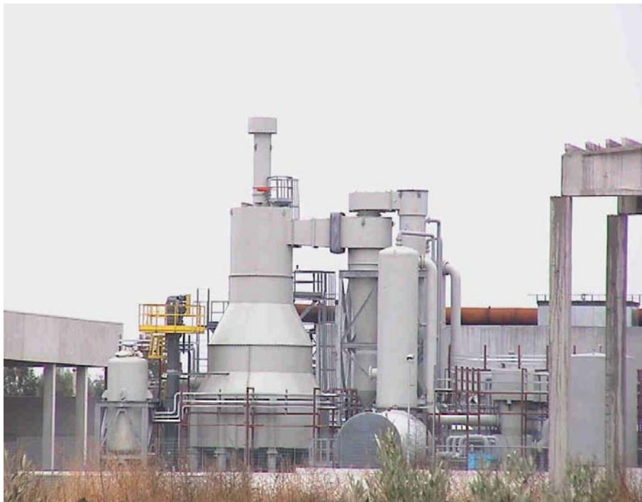
A 4 MW biomass gasification unit installed in Italy in 2001 (1/6 of proposed Selby Mine scale) 6
